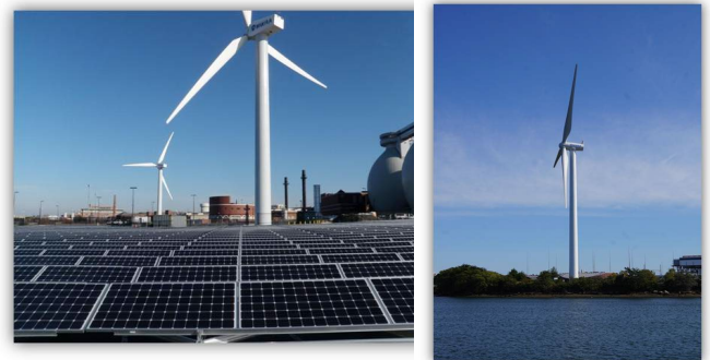
Figure 4: From left to right: Solar and Wind at Deer Island Wastewater Treatment Plant; Wind at DeLauri Pump Station
