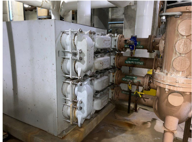
Sludge Heat Exchanger
