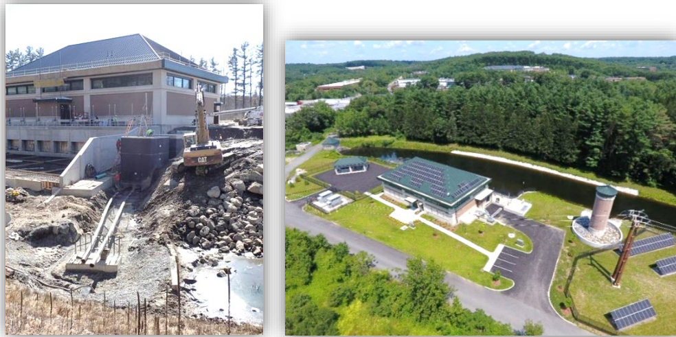
Wachusett Aqueduct Pumping Station Geothermal Heat Pump Installation
