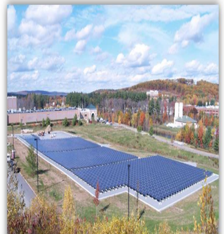
Solar at Carroll Water Treatment Plant
