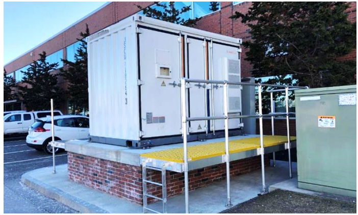
250kW Battery Demonstration Project at Chelsea Administration Facility
