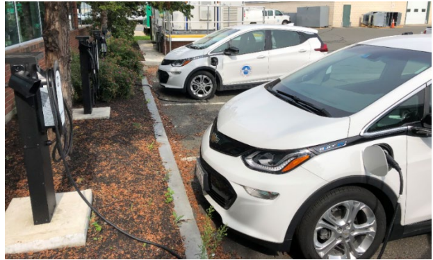
EV charging at MWRA Chelsea Facility
