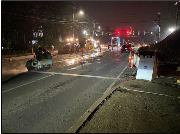
Night Work at the Intersection of Lexington Street and Totten Pond Road
